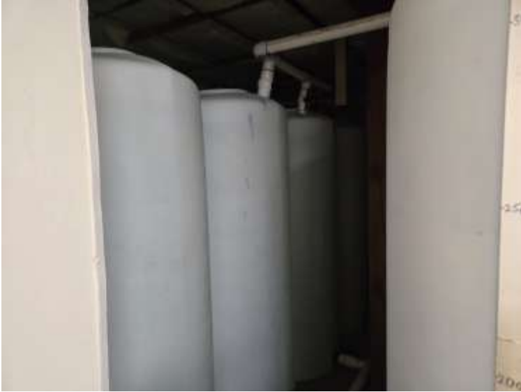
Picture 2: Upgraded Water storage system
