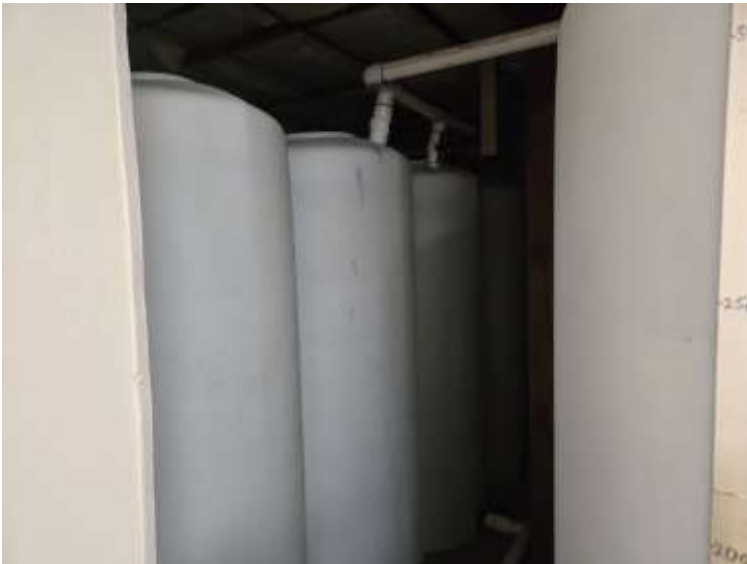
Picture 2: Upgraded Water storage system
